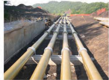
Power Plant Scrubber Pipe
