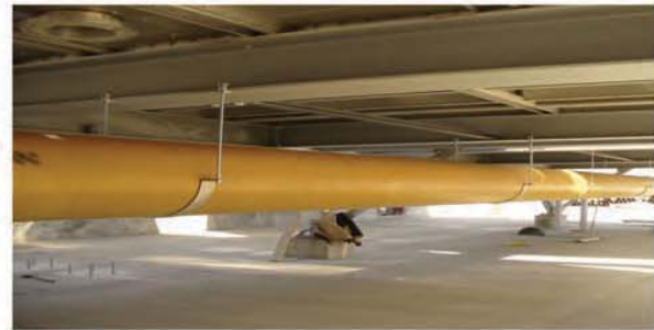
Hot/Cold Circulating Water Lines
